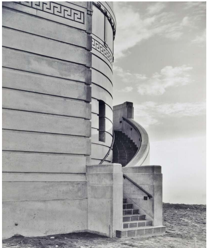
Figures 6 & 7: The west side exterior stairs during the construction of Griffith Observatory in August, 1934 (Austin-Chalk Collection, Griffith Observatory).
